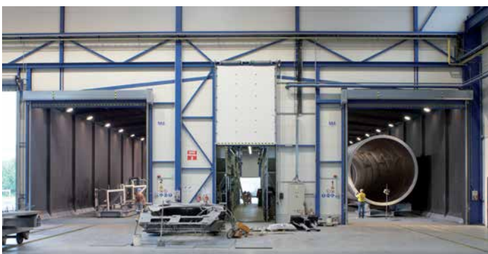
Two identical blast rooms with center-mounted machine room
