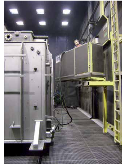
Blast room with swivelling platforms for blasting of transformers
